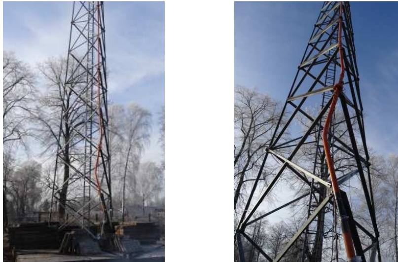
Fig. 3. Buckling of the leg in section S-7 of the tested tower – general (left) and detailed (right).
